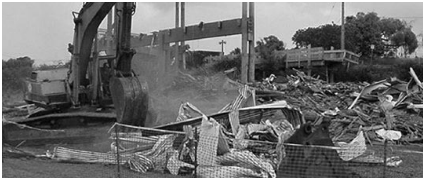
Demolition and clean-up of the old Molokai Recreation. Site was cleaned to make room for new community facility.
