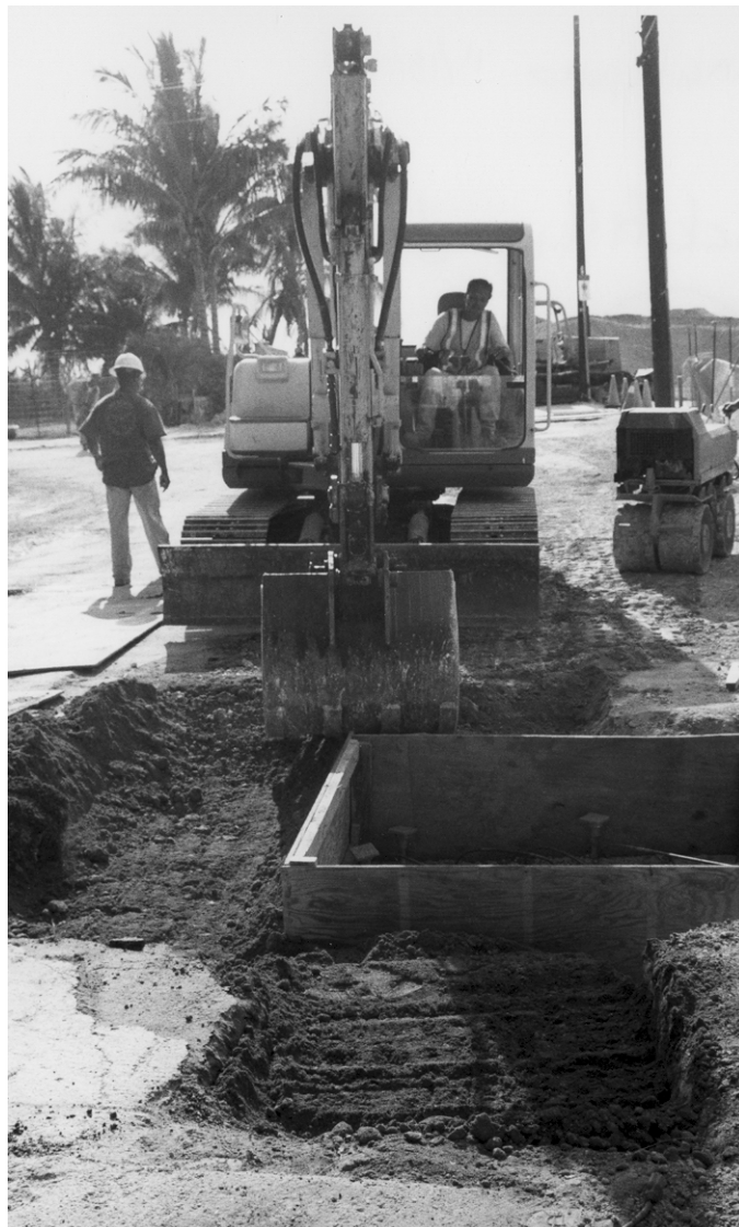
The Nanaikapono Subdivision Upgrade project provides infrastructure improvements to the roadway, drainage, sewer, water and electrical systems to one of Nanakuli's oldest subdivisions.
