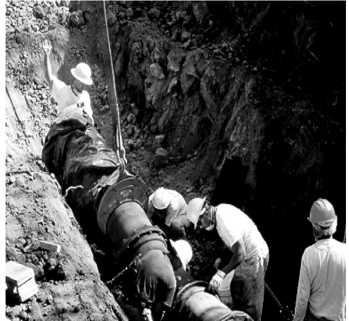
The Kula Water Transmission Main project was completed in August 2003. It provides water service to the 320 homestead lots in Waiohuli, Maui
