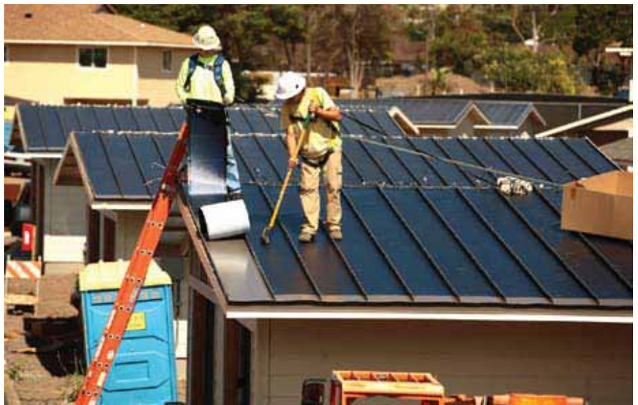
M. Watanabe Electrical Contractor workers at the Kalakaua Community, an Actus development at Schofield Barracks
