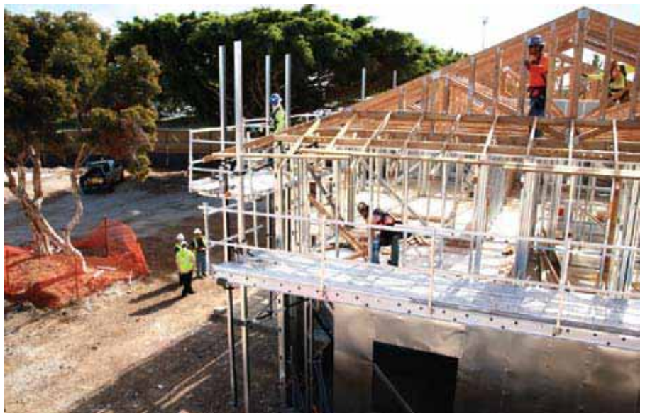
Worthington Construction is the general contractor for Actus Lend Lease’s Onizuka Community at Hickam Air Force Base.
