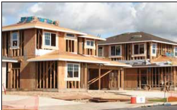
The five home plans in the Kānehili subdivision offers energy efficiency as a central theme.
