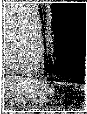
Photos 15: Showing damage to the jamb of the door leading to the pool area.
